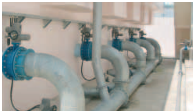
AUMA part-turn actuators mounted to butterfly valves in a Vietnamese water treatment plant.
